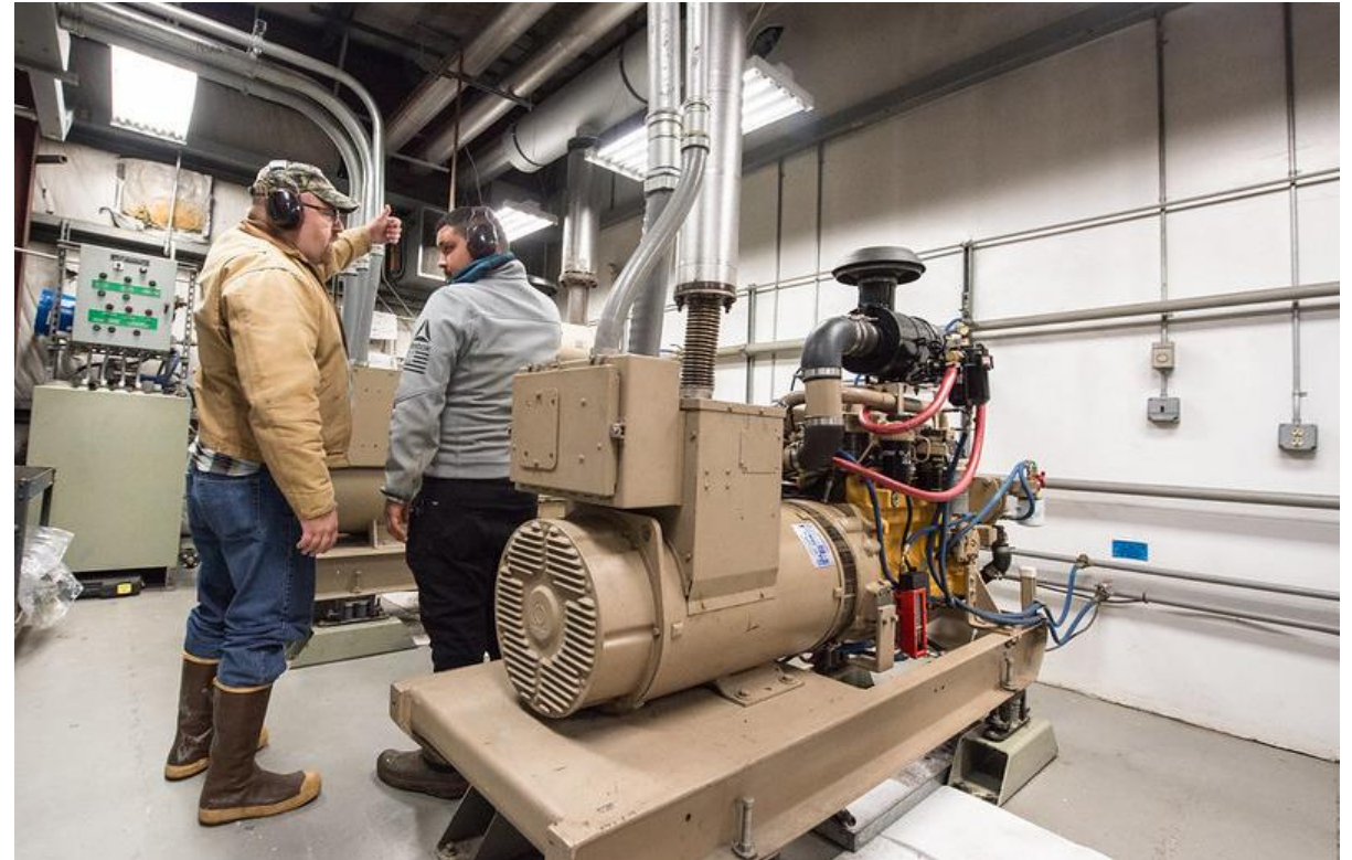
Daniel Rich, Mayor of Ouzinkie, leads a tour of the Village off Ouzinkie on Kodiak, Alaska . Diesel Power Plant. (Dennis Schroeder / NREL)
